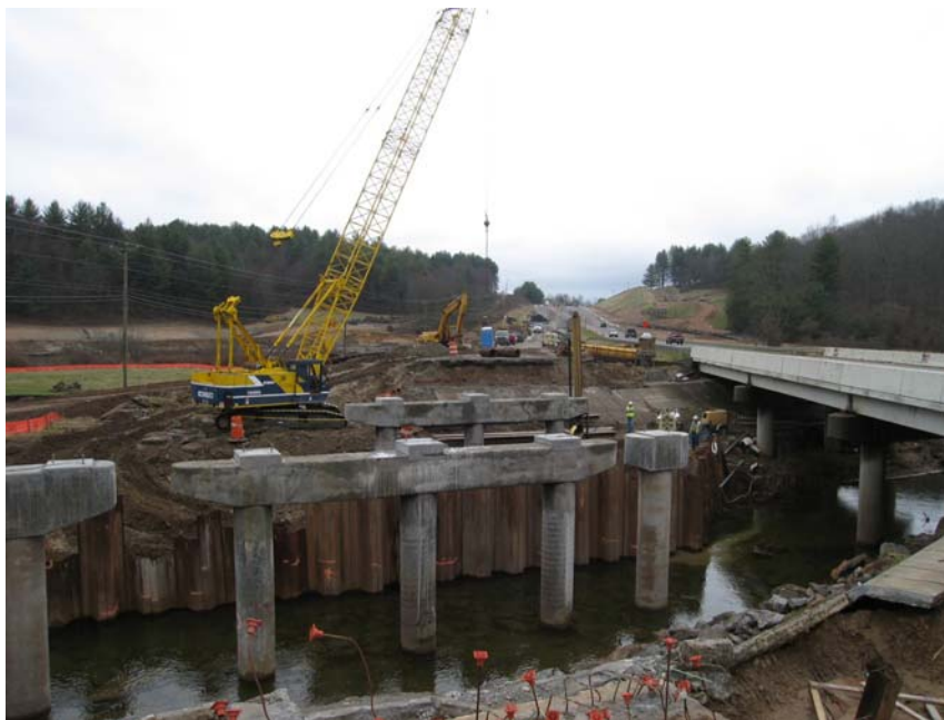
Image 2 - Area 2, B-617 cofferdam constructed to work on Pier #1 (far), Pier #2 complete (near) (3-27-09)
