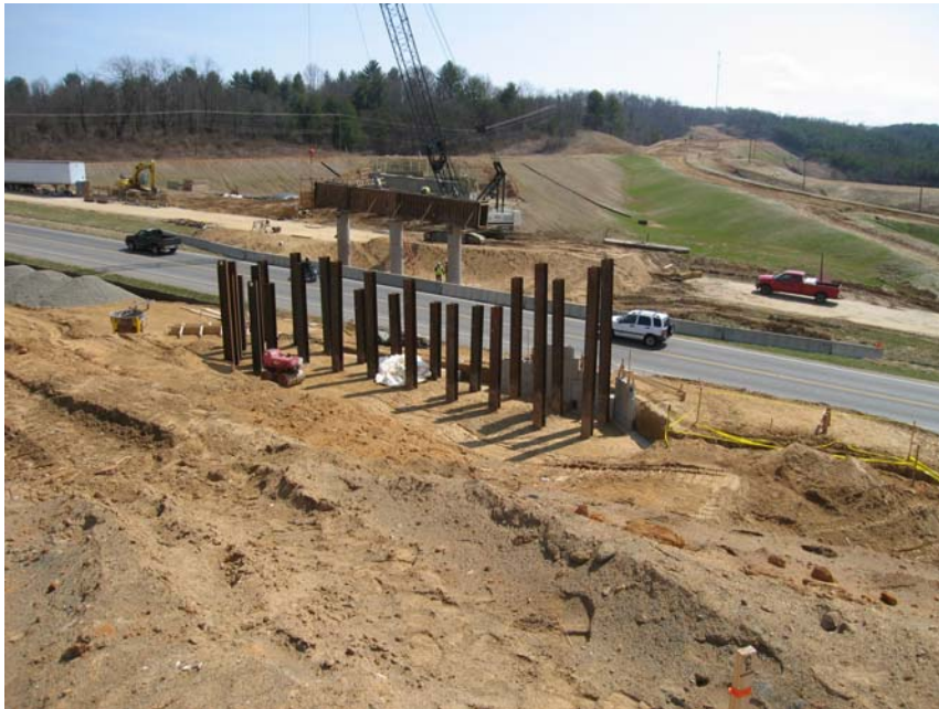
Image 4 - Area 3, B-616 Abutment A (near) H pile and MSE wall, looking east (3-24-09)
