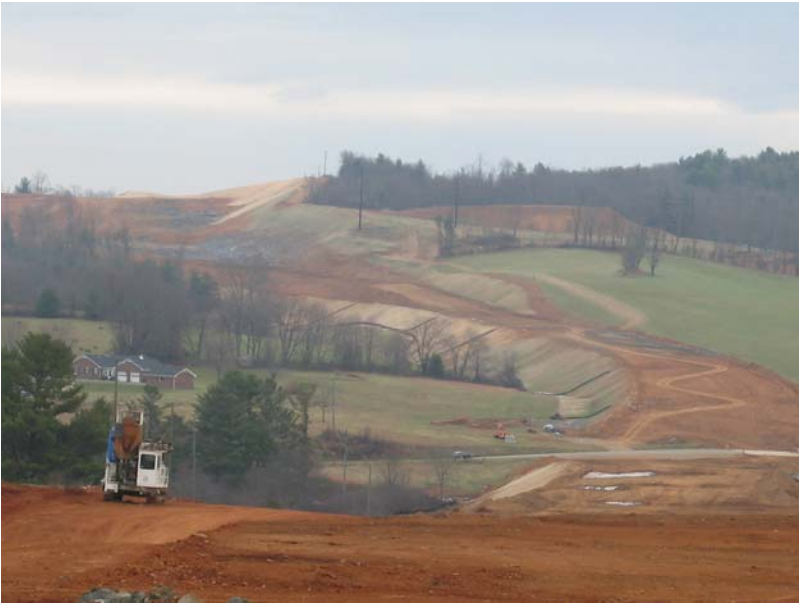
Image 7 - Area 5/6, Looking East, Fills next to Snake Creek Road (near) to Cut 6 (far) (11/24/08)
